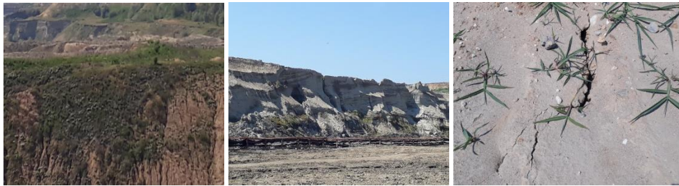
Figure 6. Gullies and ravines (left), sufosis phenomenon (middle), cracks (right)
