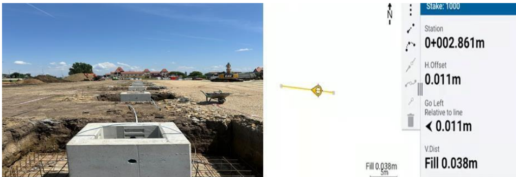
Fig. 6 Axis stakeout using stakeout line method in order to determine the center of the prefabricated structure
