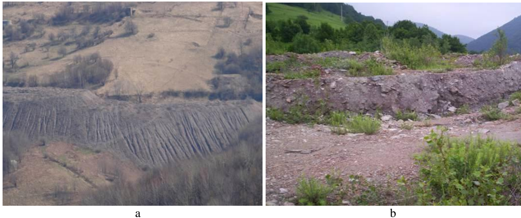
Fig. 2. Slope erosion and uneven settlement of upper platform
