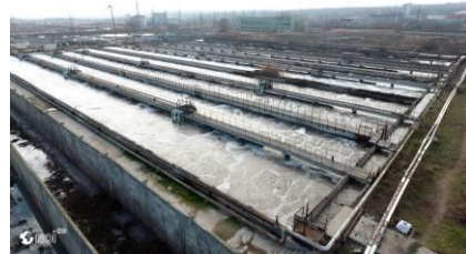
Fig. 8. Chișinău wastewater treatment plant - filters
