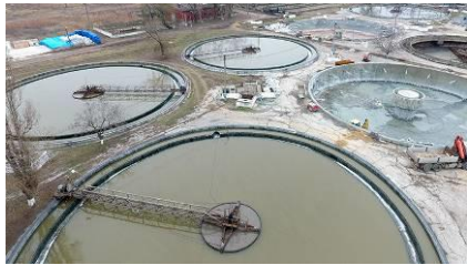
Fig. 7. Chișinău wastewater treatment plant - decanters
