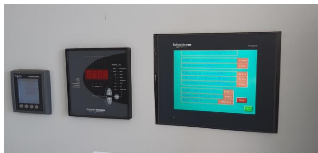
Photo 9 Pump control panel display
